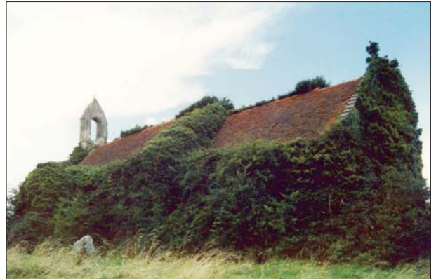
▲ St Denis', East Hatley in 2003, covered in ivy and in danger of collapse.
